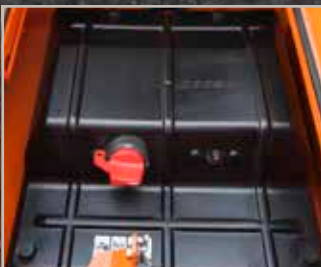
Battery cut-off switch
